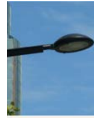
FIGURE 16: LIGHTING FIXTURES ADAPTED FOR PEDESTRIANS
