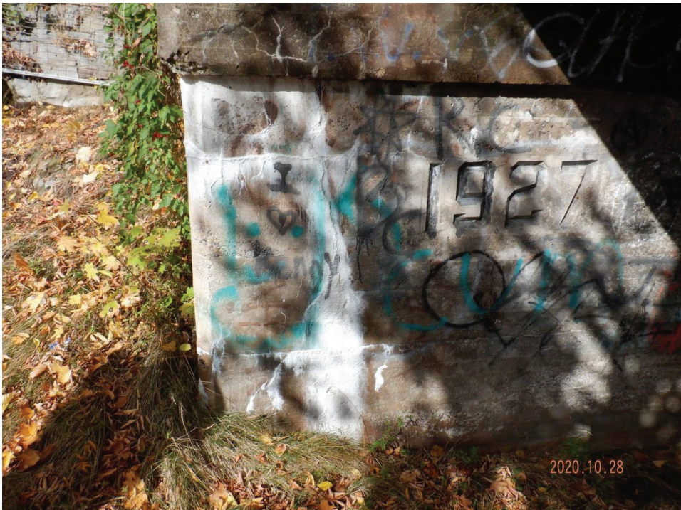
Cracking with efflorescence in northwest abutment wall
