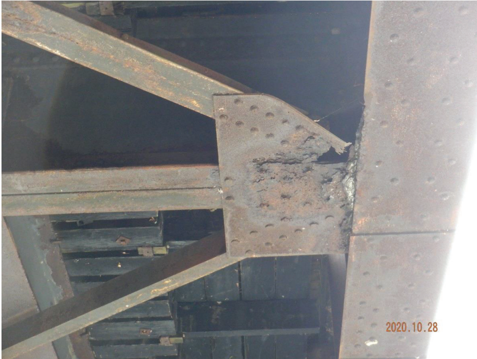
Perforation in south gusset
