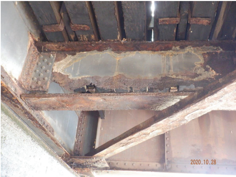
Perforation in northeast stringer
