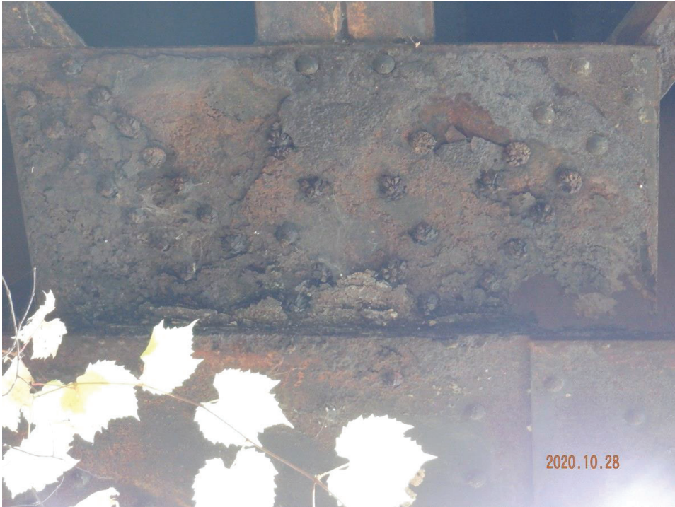
Perforation northeast gusset plate
