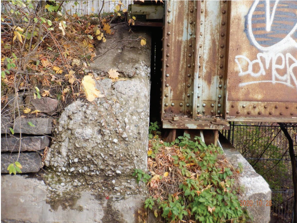
Disintegration in northwest ballast wall
