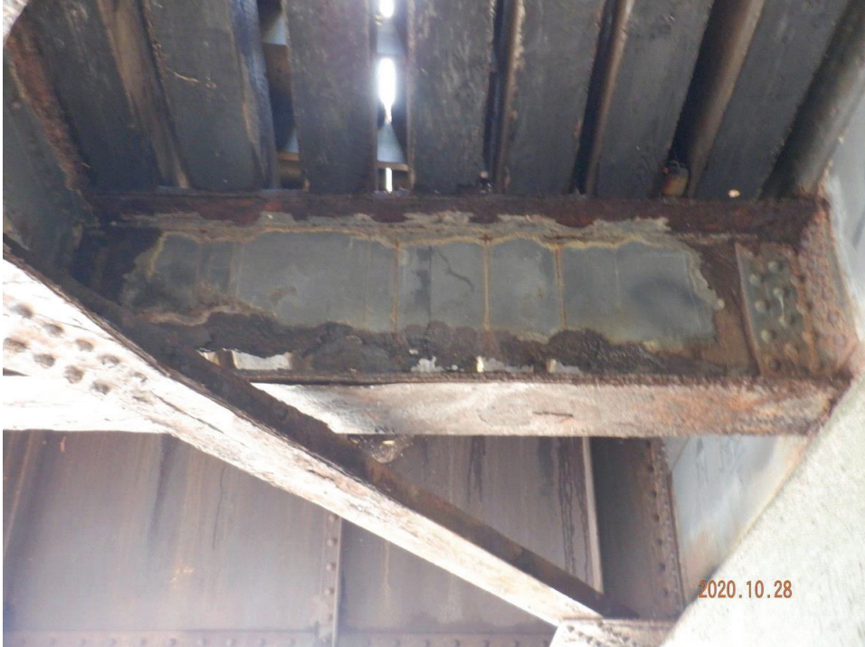
Perforation in northwest stringer
