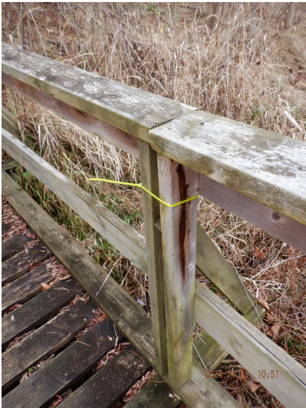
Figure 10 : Bridge Railing-Evidence of Loose Connection
