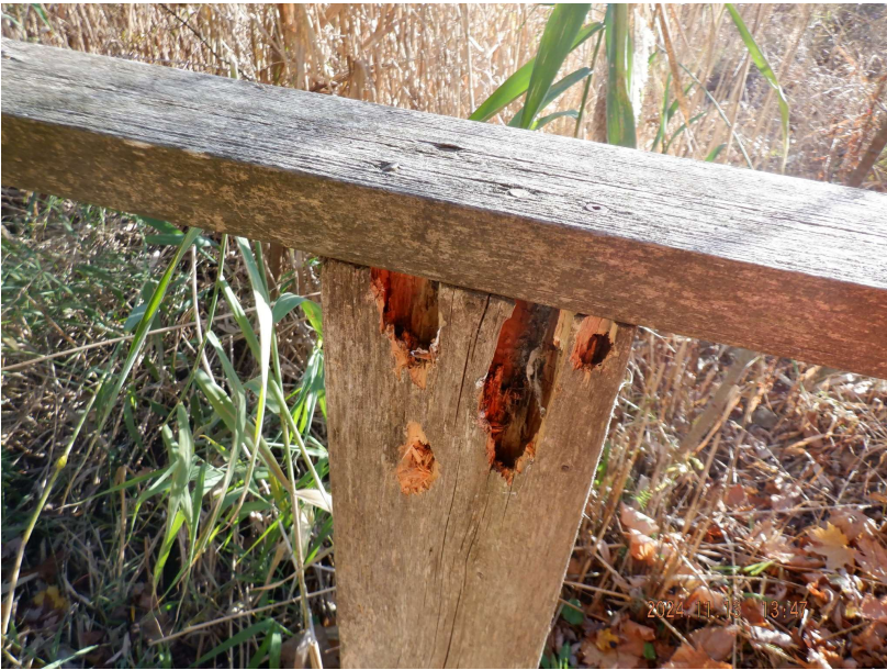
Figure 9 : Railing-Evidence of Severe Rot
