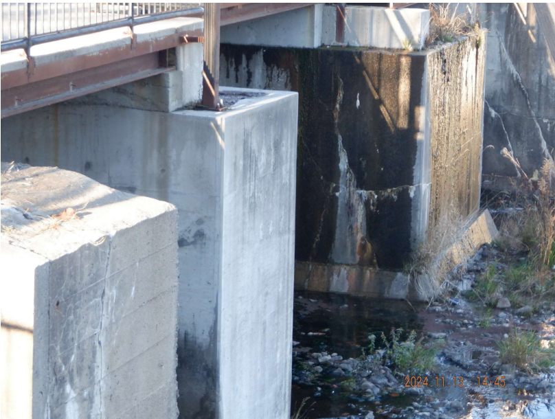
Figure 18 : Dam Sluits (Typ.)-Evidence of Wide Crack with Efflorescence
