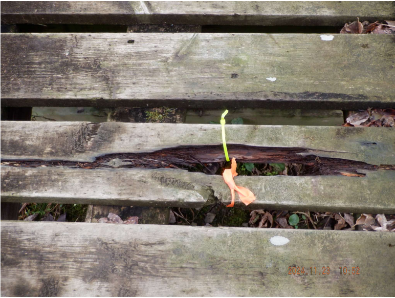
Figure 12 : Bridge Deck-Broken Plank
