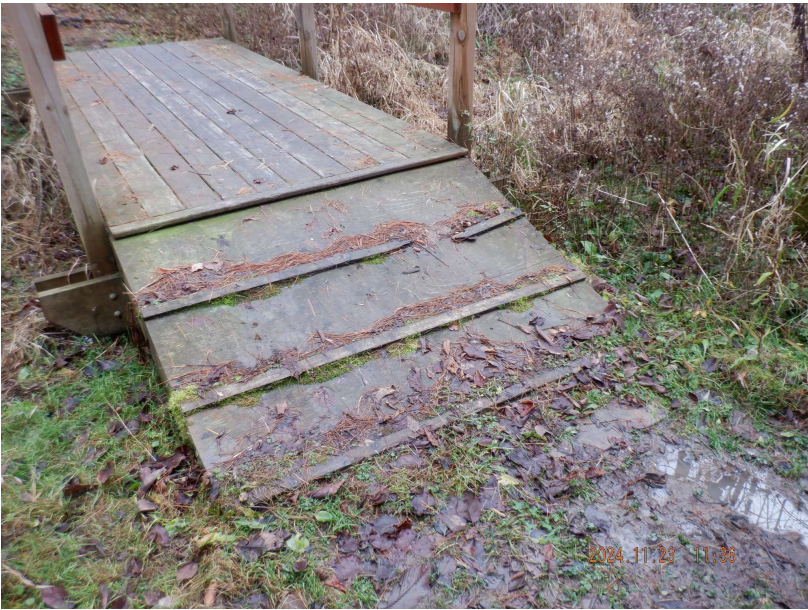
Figure 5 : South Ramp-Evidence of Broken Timber & Localized Failure of Ramp Ribs
