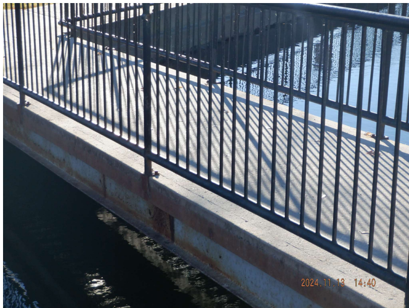
Figure 10 : Exterior Railing & Fascia-Evidence of Medium Rust
