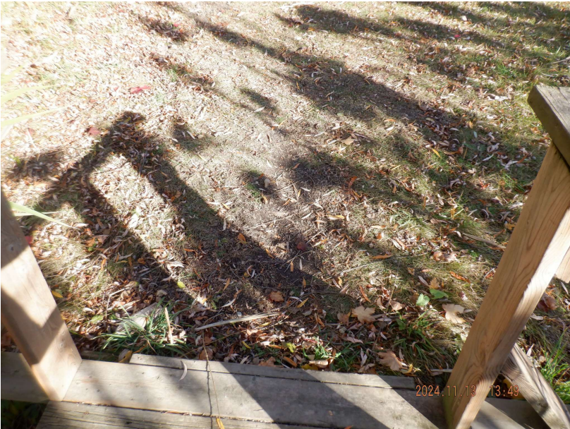
Figure 14 : East Approach-Evidence of Tripping Hazard
