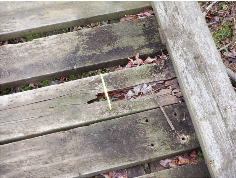
Figure 11 : Bridge Deck-Broken Plank
