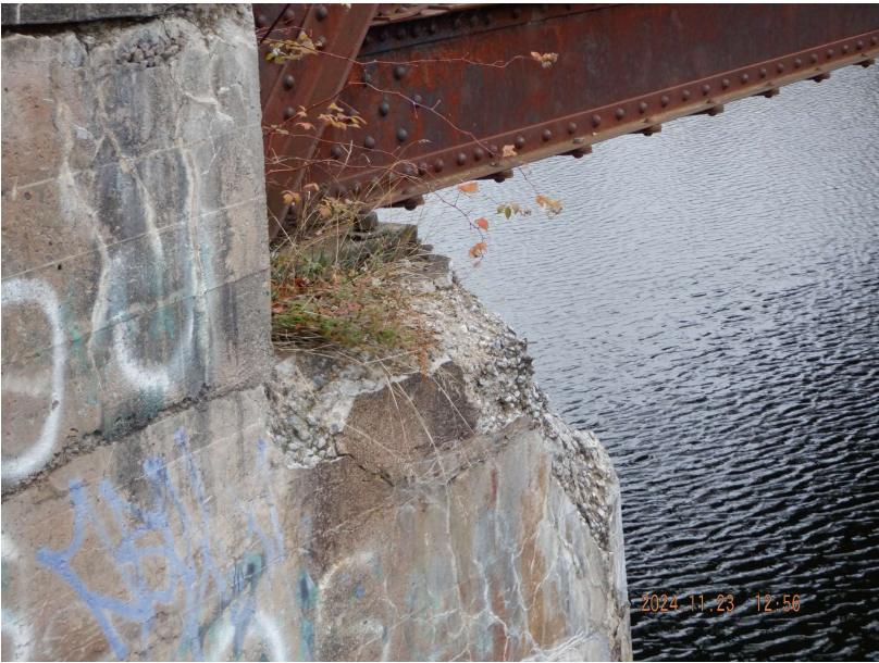
Figure 11 : Bridge Bearing Seat (Typ.)-Evidence of Severe Disintegration
