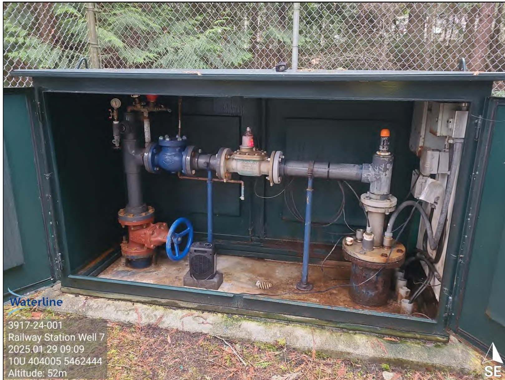
Photograph A7: RSW 7 – Looking inside the well house. Leaky wellhead fitting noted causing some corrosion of the casing lid.
