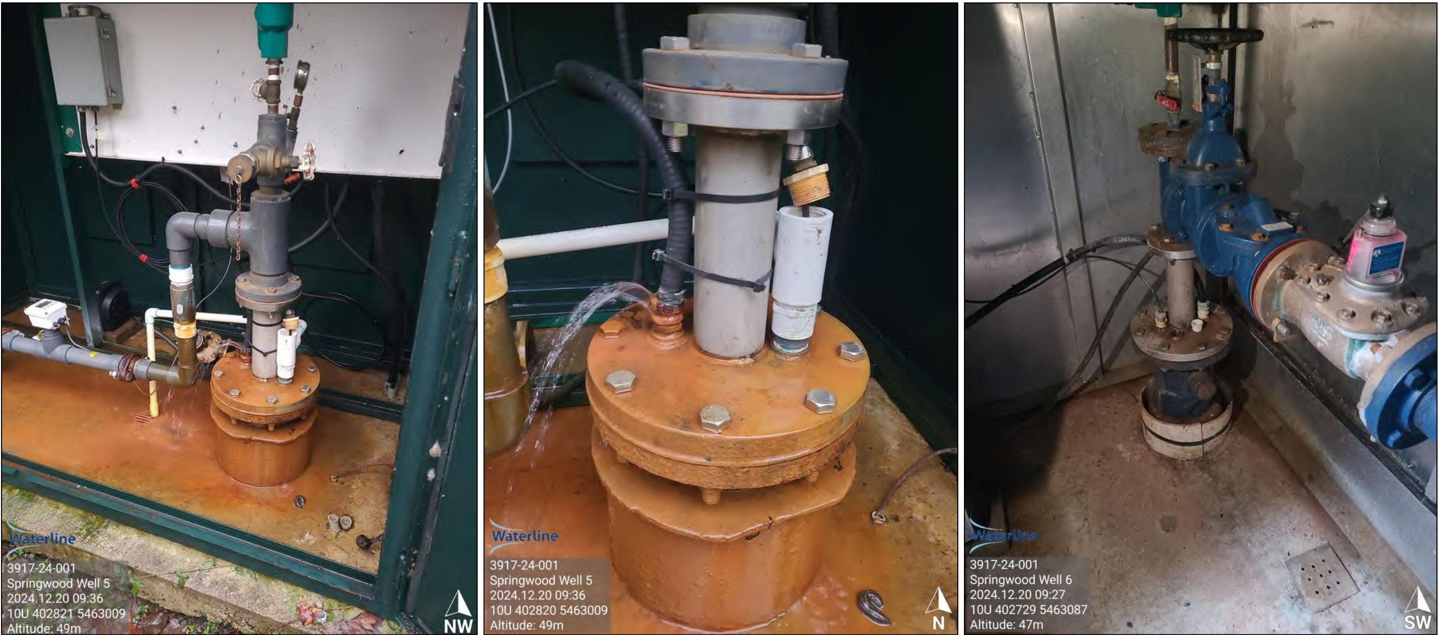
Photograph A13 (LEFT): SW 5 – Looking inside the well house. The well is flowing artesian during periods of non-pumping. Photograph A14 (MIDDLE): SW 5 – Close-up view of the wellhead. The pressure fitting for the electrical cable to the pump is leaking, allowing for uncontrolled flow and standing water to accumulate in the well house. As a result the wellhead components are corroding, leading to iron staining (oxidation) and bioaccumulation. Photograph A15 (RIGHT): SW 6 – Looking inside the well house. No issues noted.
